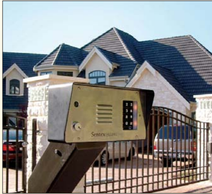
AVD Media's installation consisted of security, including intrusion detection and biometrics, automatic lighting control and home theater, and more.
