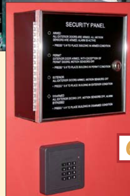
6. A locked security panel with an Arm/Disarm display resides above one of 17 HID proximity readers included in the project.
