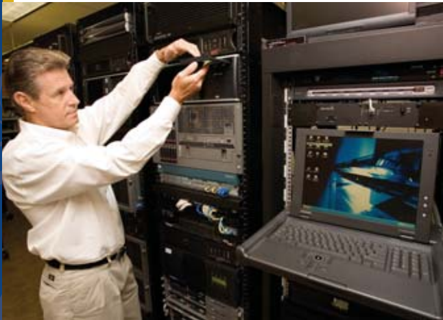
HSM Operations Manager Keith Kilpatrick inserts a CD into one of four Honeywell DVRs located in Silver Eagle's main IT hub and equipment room. The video surveillance system includes more than 50 Bosch cameras.
