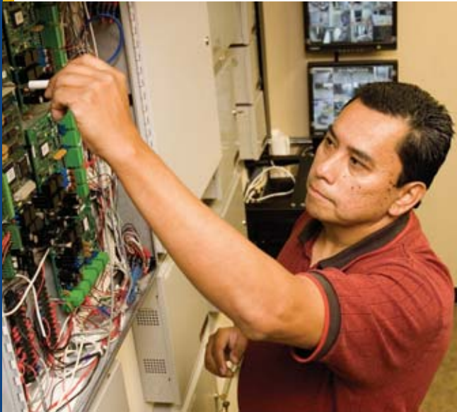
HSM Field Installation Specialist George Osorio tinkers with the inner workings of a control panel located in Silver Eagle's main IT hub and equipment room. The system includes 53 points of intrusion protection and 32 access control card readers.
