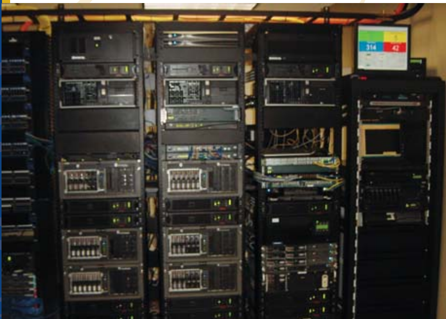
This wall of equipment racks is located in Silver Eagle's main IT hub and equipment room. It includes components for the video surveillance, access control and intrusion systems.
