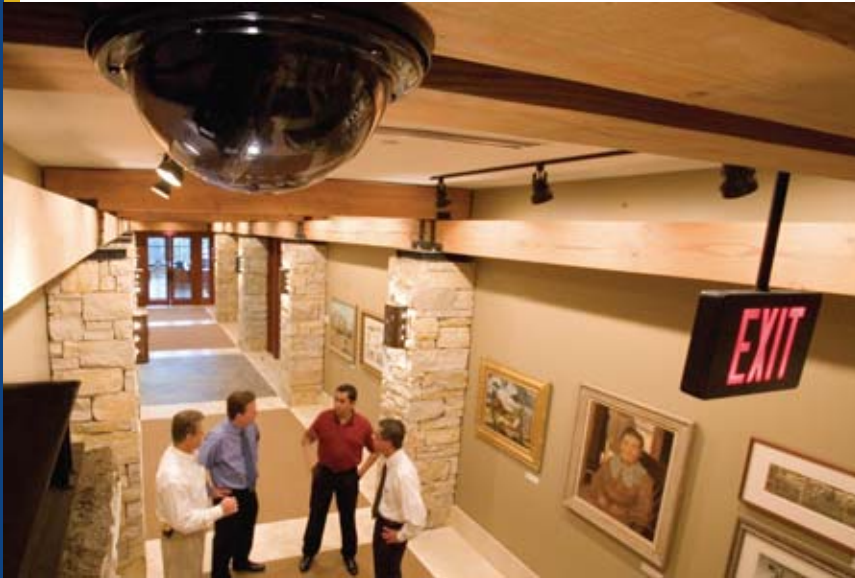
An area dubbed the "Walk of Fame," which features many fine pieces of art, required some special handling on the part of HSM. The finished construction in the hallway has exposed beams similar to a rustic hunting lodge and so all wiring had to be well concealed, with cameras and motion detectors as unobtrusive as possible.
