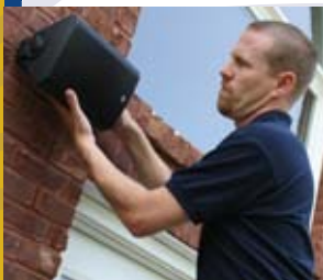
Life & Property Security Systems Technician Lee Rowland mounts one of the outdoor speakers connected to the whole-house audio system.
