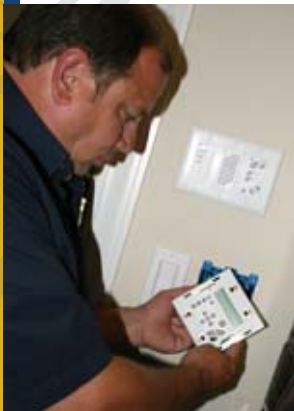
Life & Property Security Technician Robert MacAuley puts the finishing touches on installing a Russound audio keypad in the kitchen. The Greyfox master intercom station can be seen on the wall in the background.
