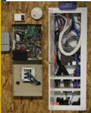
Here we see the inner workings of the home's structured wiring, security, lighting and intercom controls, which were mounted in one location to allow easier integration and maintenance.
