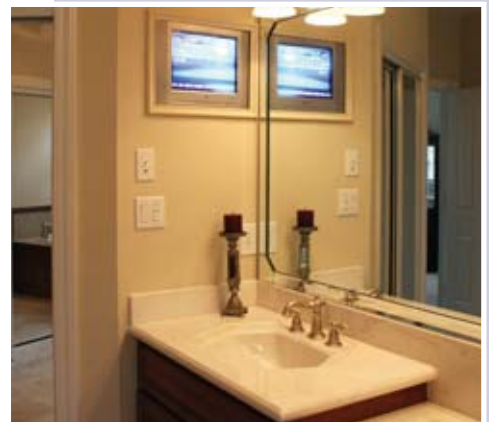
Television monitors, which can also be used to view CCTV cameras, are located throughout the home, including this in-wall bathroom installation.
