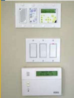
The top control is a Russound audio keypad combined with a Greyfox intercom unified via a custom wall plate to reduce the required wall space and create a sleeker appearance. Also pictured is a X-10 Pro light switch and a Honeywell security system keypad.
